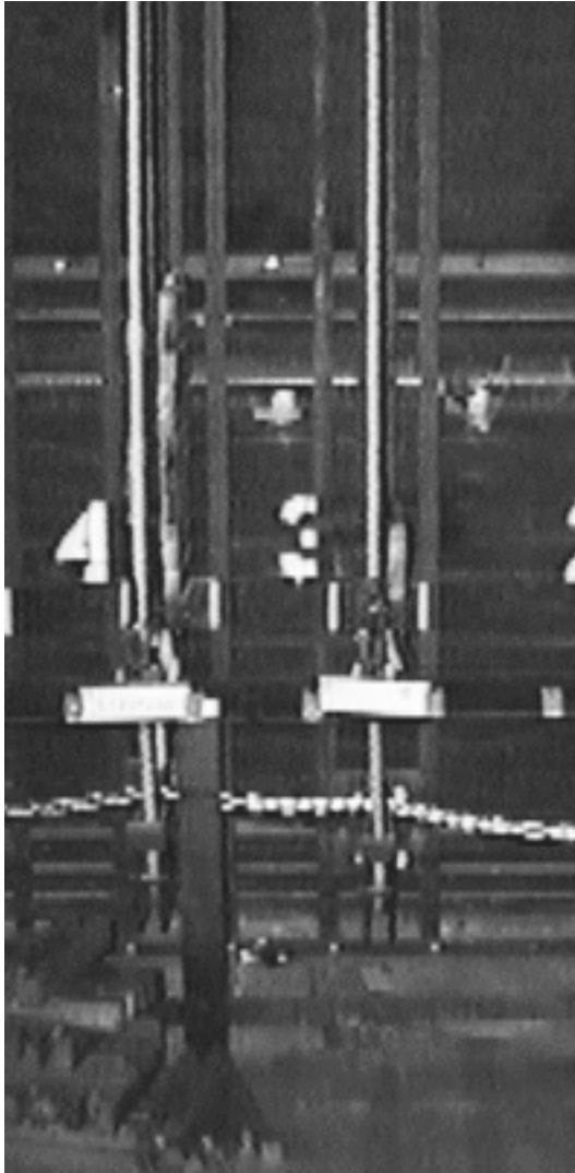
Figure 4.6: A portion of the counterweight fly system in Alden Hall at WPI.
